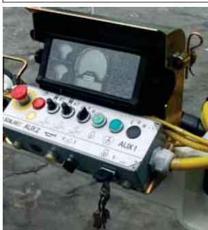
DRILLING CONTROL BOARD
